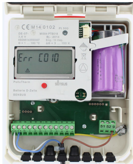
Figure 10: connected Flow sensor
